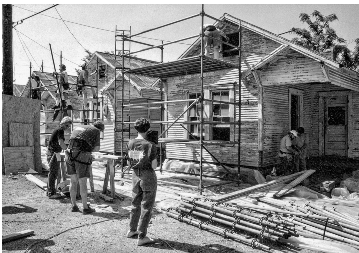
Amoco employees from across the United States participating in the first large-scale volunteer effort at Project Row Houses , organized by Amoco Torch Classics, a program for the corporate Olympics. This effort renovated the exteriors of sixteen houses in 1994. Photograph courtesy of Project Row Houses .
