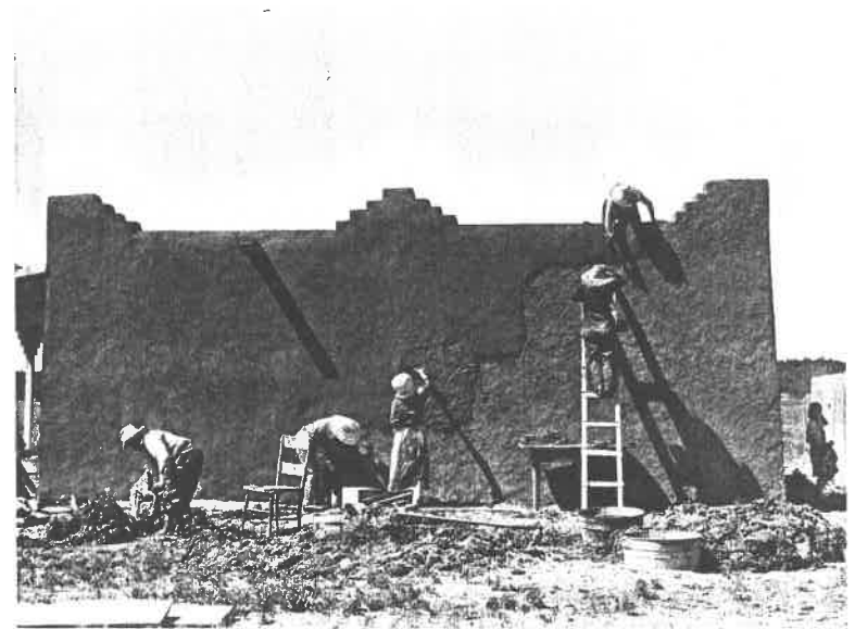
2.8 Dwellings and social reproduction. Rural vernacular architecture and the building process: house in Chamisal, New Mexico, receiving a new application of adobe by local women, 1940. (Photograph by Russell Lee, Library of Congress.)
